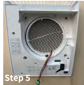
Step 5 Push heat recovery and fan cartridge into PVC pipe (photo w.o. filter) for final wiring and connection.
